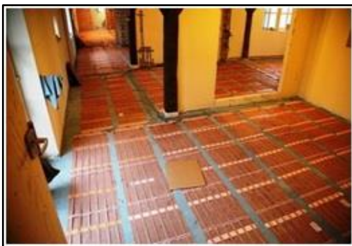
Floor heating in a farmhouse
